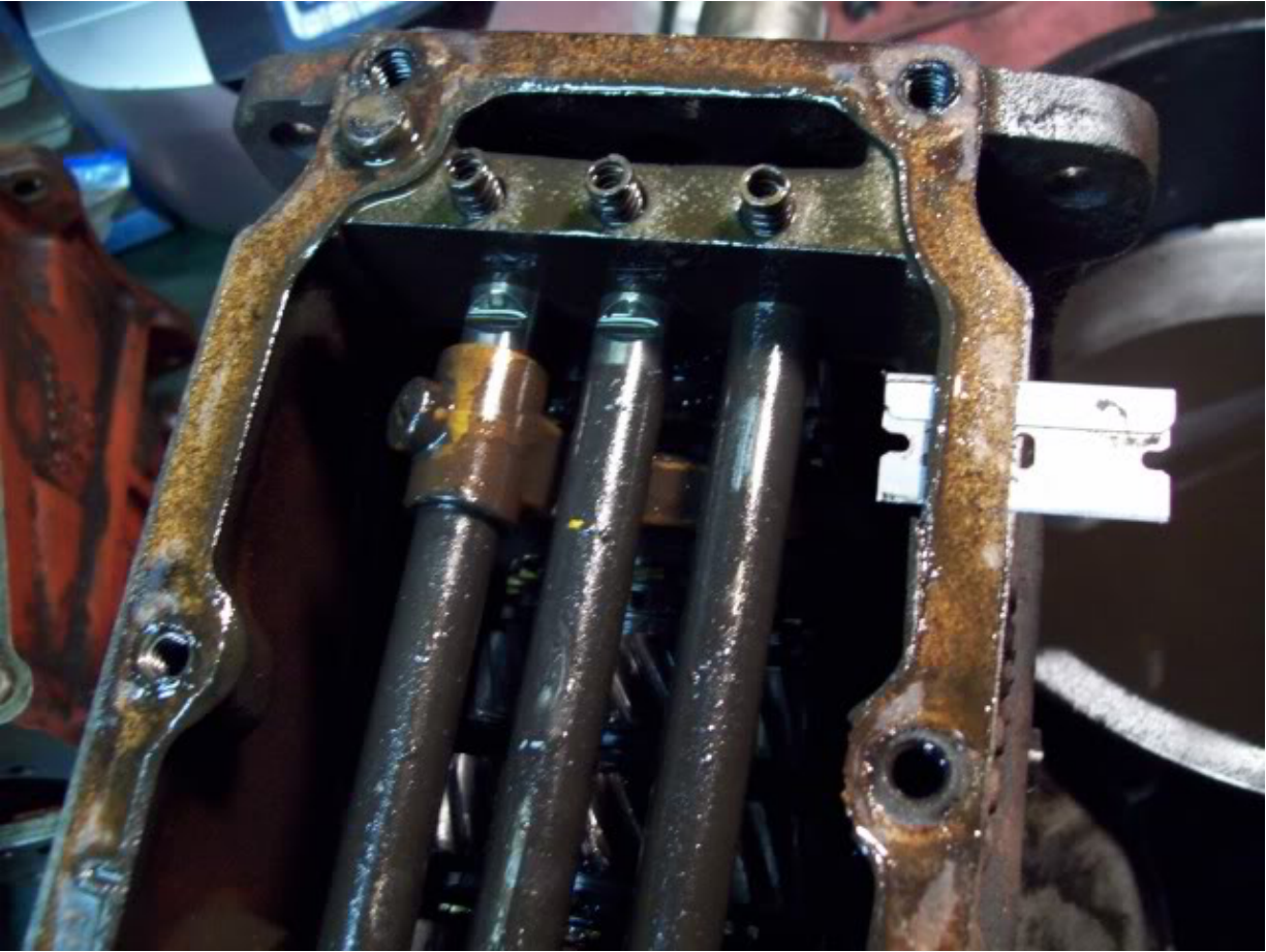
We can see the damaged gear from here:
